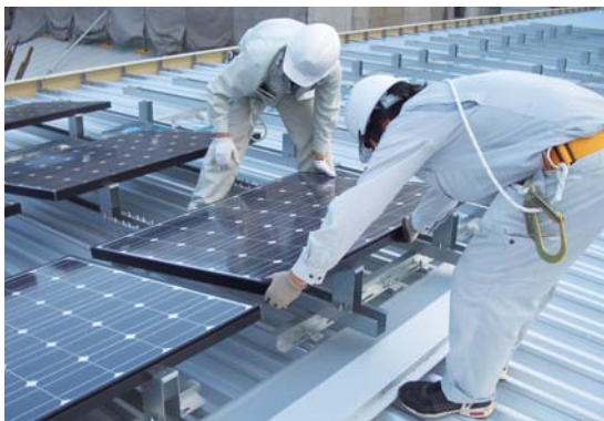
● Scene of the installation of photovoltaic power generation system
