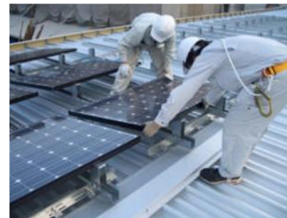
Installments of solar power systems
